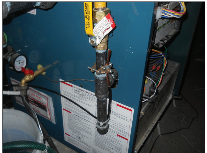
Example of Bonding at the Drip Leg
