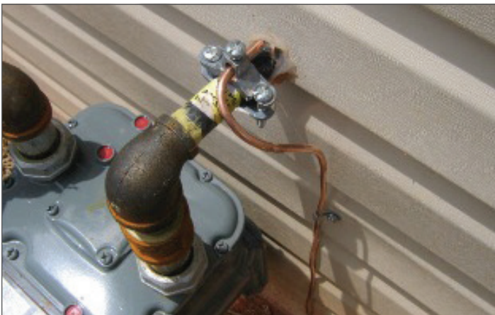
Example of Bonding at the Service Entrance
